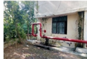
WET ALARM SYSTEM
