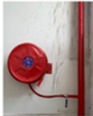
HOSE REEL SYSTEM
