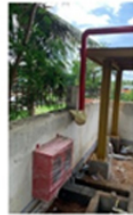
HYDRANT VALVE HYDRANT BOX
