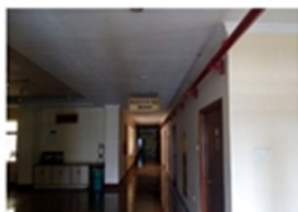
SIDE WALL SPRINKLERS & FIRE EXTINGUISHERS
