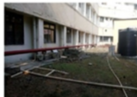
EXTERNAL HYDRANT LINE
