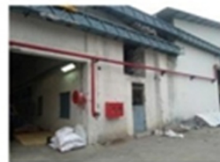
HYDRANT VALVE, HOSE BOX & HOSE REEL DRUM
