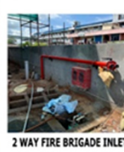
2 WAY FIRE BRIGADE INLET
