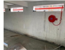
HOSE REEL AT PARKING
