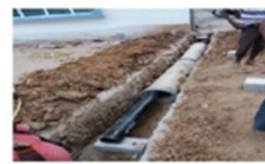
UNDERGROUND PIPING WITH WRAPPING & COATING
