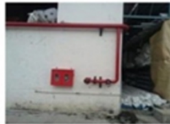
2 WAY FIRE BRIGADE INLET
