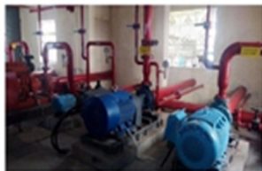
ELETRICAL + DIESEL + JOCKEY FIRE PUMP
